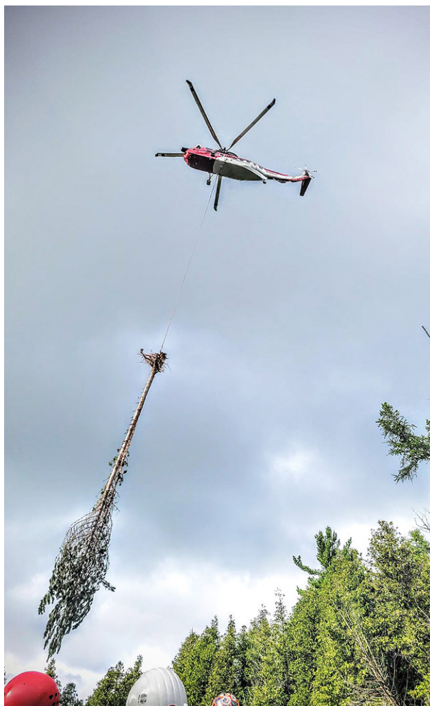
Construction Helicopters pilots position a pine tree before dropping it in the Manistee River.
