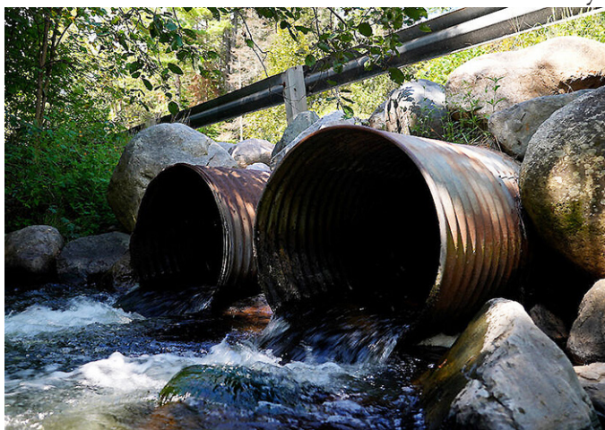
Road and stream crossings often have culverts like this that restrict upstream access for aquatic organisms and most importantly trout. Trout Unlimited photo.
