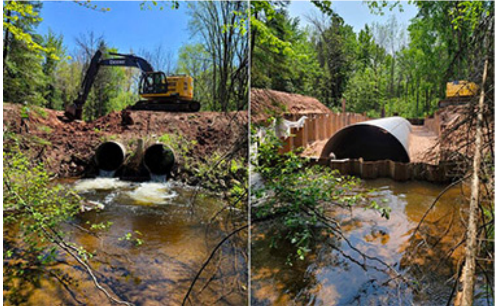
Left: Two perched, undersized culverts on Trout Creek blocking fish passage; Right: the new properly sized structure getting installed on Trout Creek
